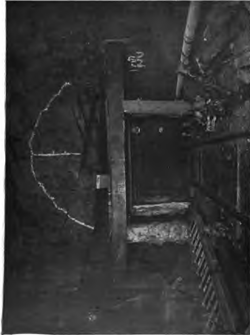
PLATE 200.—Excavation of Tunnel by Bottom Heading Methods. Timber platform in position to receive Muck from upper half which is drilled from platform and blasted by use of horizontal holes placed near painted line on perimeter of tunnel.
